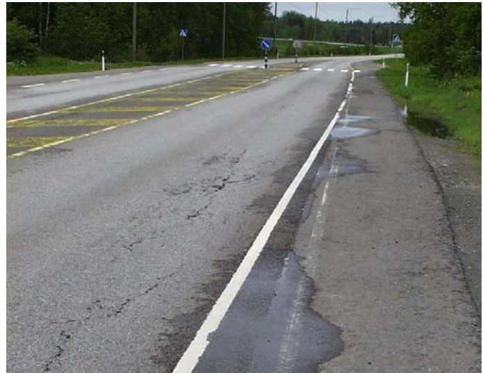
Excess water in this pavement is seeping out between the carriageway and shoulder. It's also the cause of premature pavement cracking
