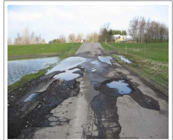
Example of an asphalt pavement distressed by being under water during the wet seasons.
