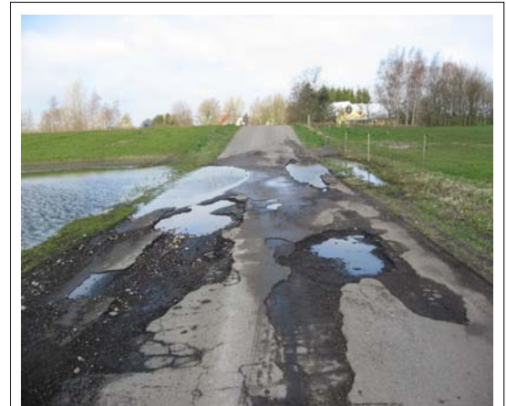
Example of an asphalt pavement distressed by being under water during the wet seasons.
